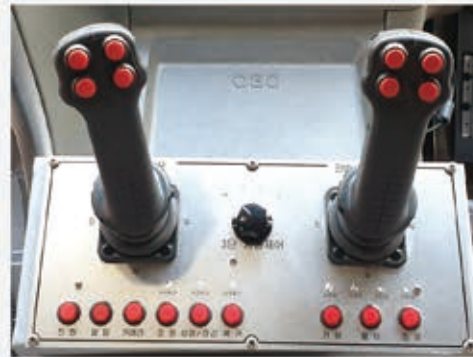
Automatic waterproof gun control panel 자동방수총 컨트롤판넬
