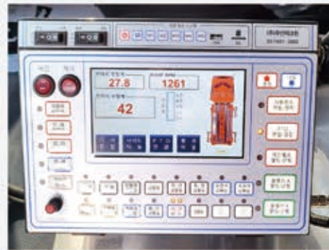
Driver's seat control panel 운전석 조작반
