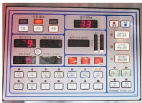
소방펌프 조작판넬 Fire pump operation panel
